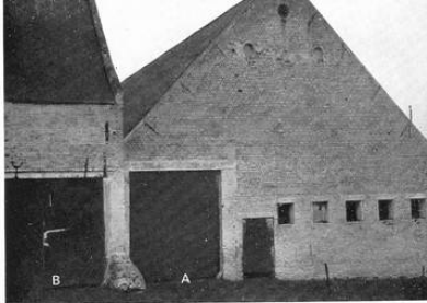
32. The entrances to La Haye Sainte from the west (the small door, right, is post-Waterloo). The door of A was burnt on the night of 17 June, so the passage was barricaded with farm machinery and French dead. B was broken into, but held by KGL riflemen (see number 31).
